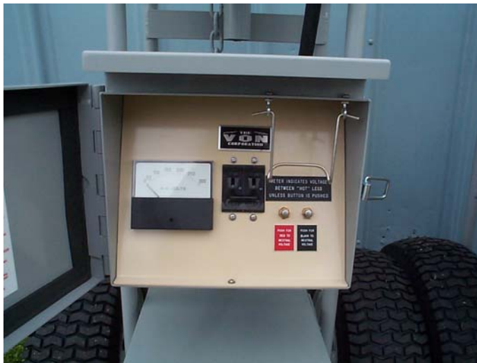
Breaker Box of Metered Unit
